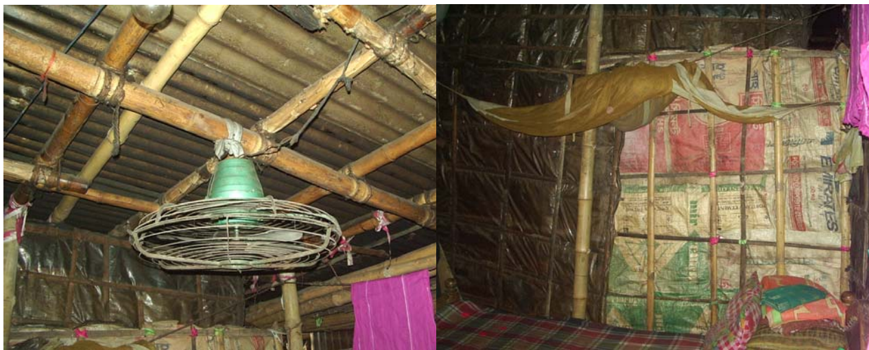
Picture 9.1.1c Construction of wall and roof with bamboo, CI sheet, plastic and hard paper (Source: Author, 2008)
