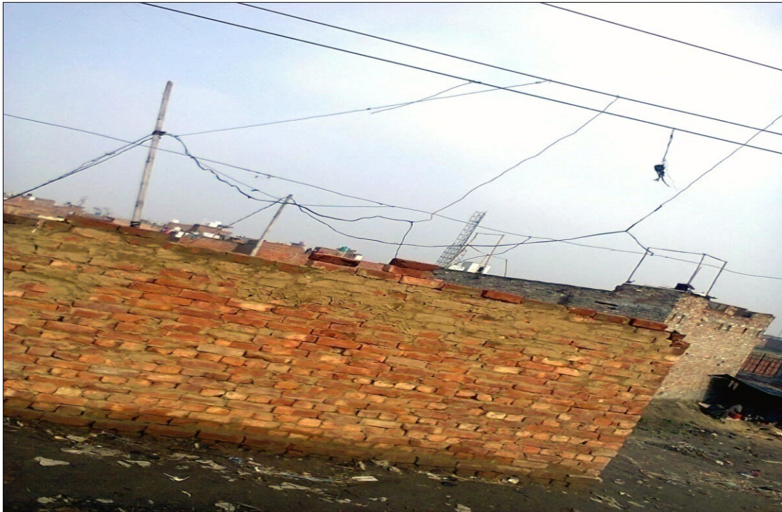
Photograph 6.2 -Electricity Theft- Dangerous and lack of provision of services in a Slum in Amritsar
