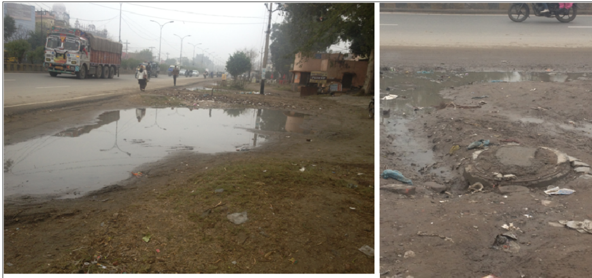
Photograph 7.2- Water Accumulation with nominal rains, Choked Sewers in
