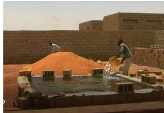
Figure (11): Construction of the core-unit core-units of Elthora hara 72 .Source : (the State Fund archives)
