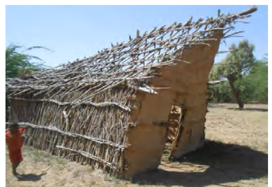
Rectangular house damaged by frontal undermining caused by standing flood water. © IOM- James Kennedy
