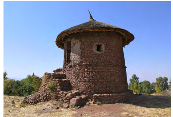
Stone tukul in Lalibela with two levels and exterior staircase. CC- Martijn Munneke
