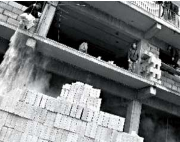
Illegal additions to existing buildings
