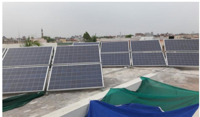
Figure 4: Solar PV system (Interview F)
